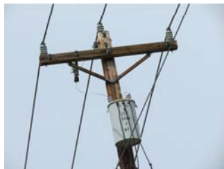
CONNECTS TO: OVERHEAD TRANSFORMER
