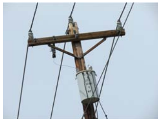
CONNECTS TO: OVERHEAD TRANSFORMER
